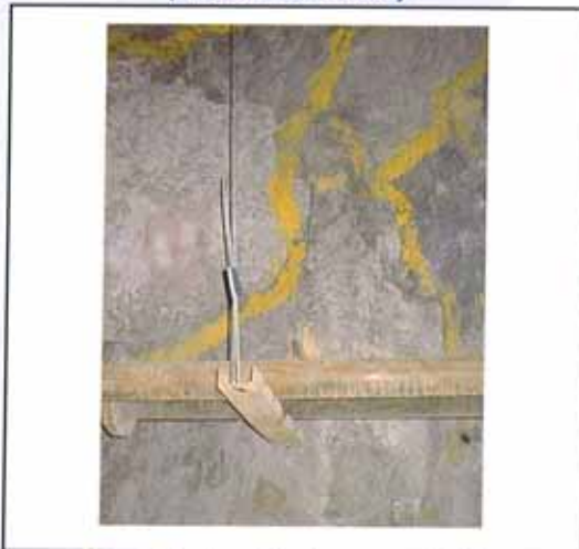
Pipe Rack - Underground Mine
